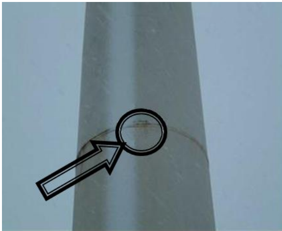
Crack in the weld of the tower
